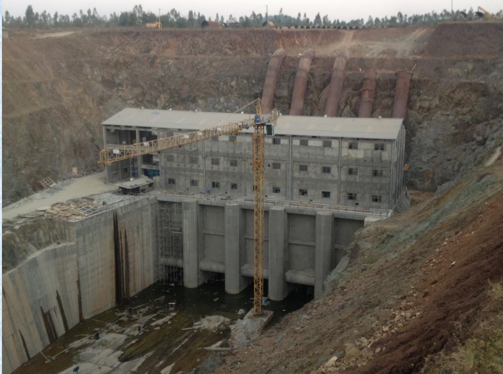
Upper Bhadra Project -Pump House near Shantipura
