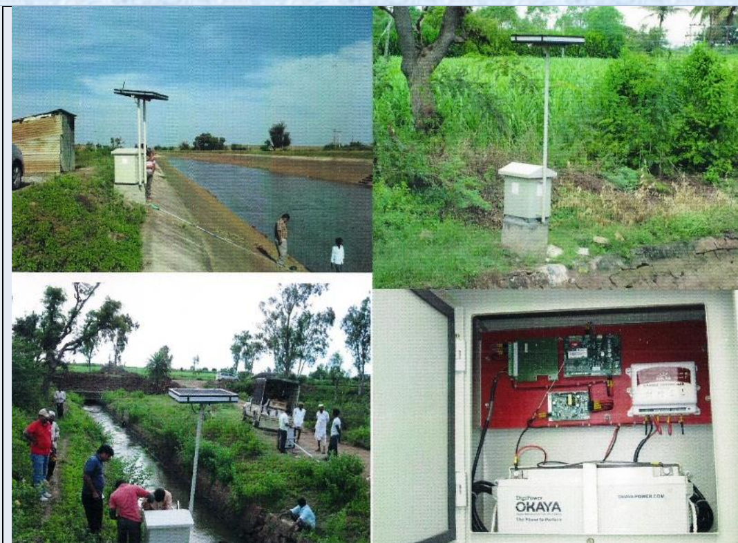
Real Time Flow measurement system
